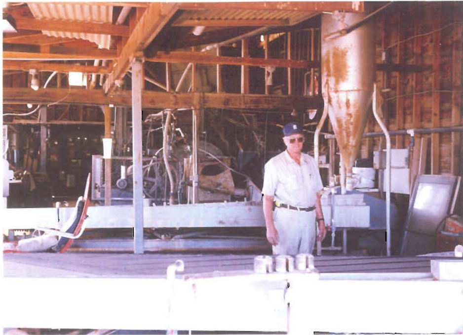
Button mill, above, with Sylvester Dimmer standing between two gravity tables with ball mill behind. Agitated vat leach tanks and carbon columns are beneath mill.
